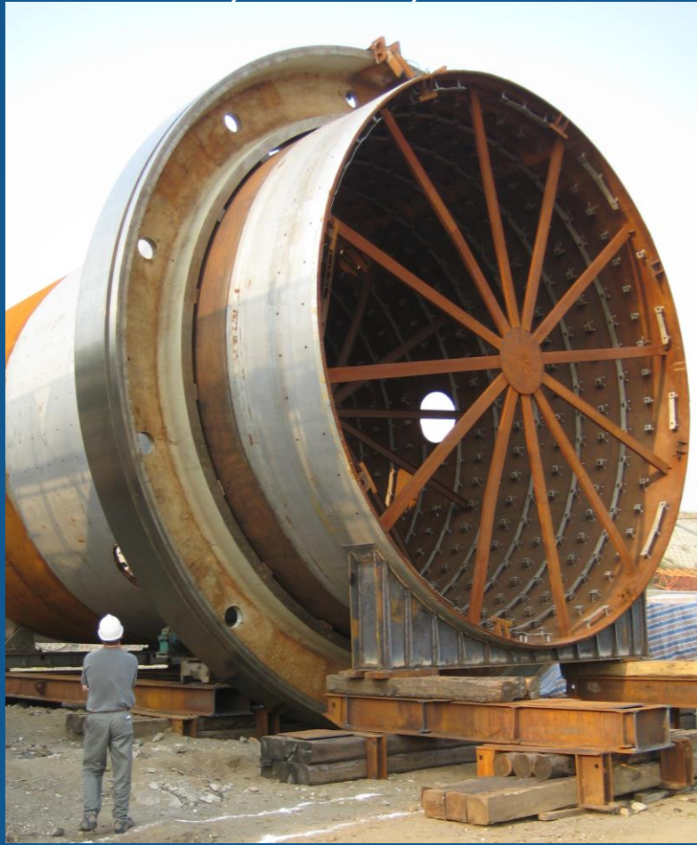
Support Tyre Placed on Outer Shell (Shell Fabricated in China, Tyre Cast in Czech Republic)
